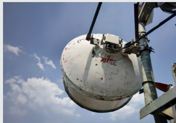
Microwave installed with additional support rod to withstand high wind pressure
